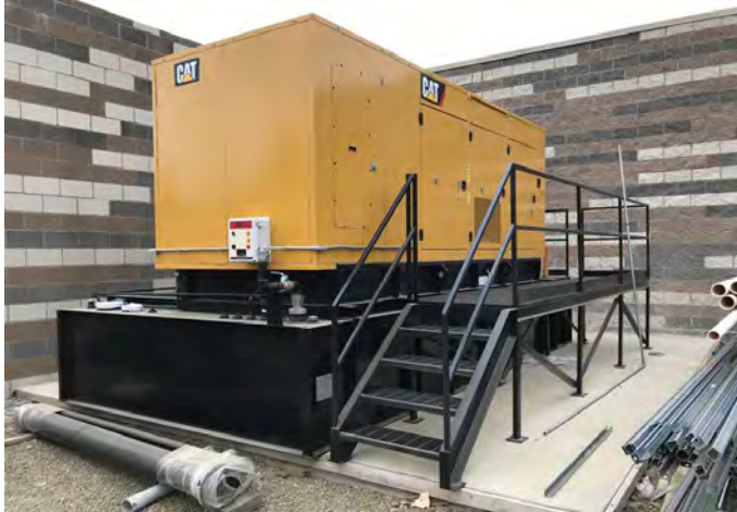
Figure 6-1: Typical stationary backup diesel generator with belly tank fuel storage.
